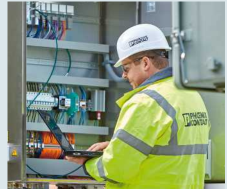
Use of the remote control and automation system in a power grid
