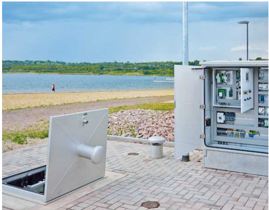
Remote control technology for distributed wastewater pumping stations
