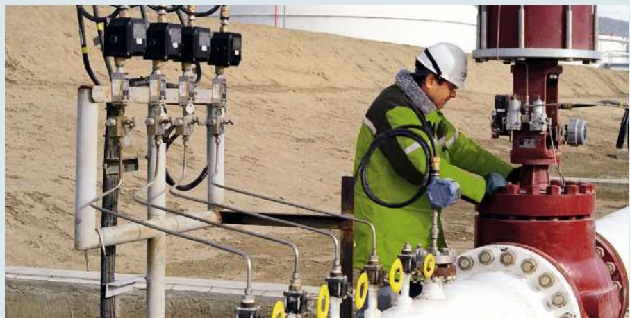
Measurement station sensors on a pipeline
