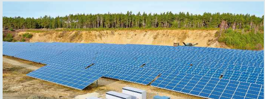
Use of a feed-in management controller in a PV power station
